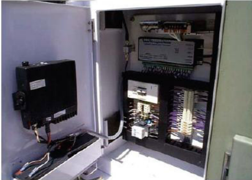
Figure 4: An HWT PDS Compact 500 RTU (similar to the one used in the Maroochy Shire SCADA)
